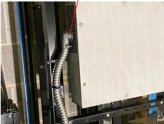
1" Flex Conduit from 90° Connector at Car Top Box
